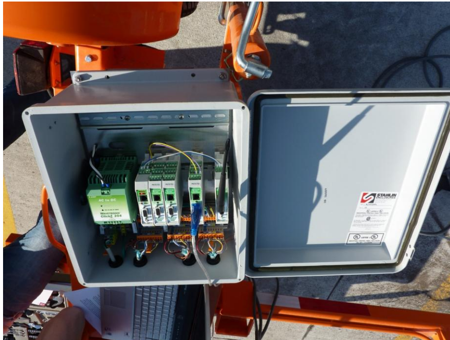
Figure 3.12: Portable sensor pole cabinet
